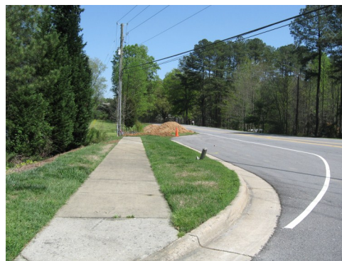
Sidewalk construction on the north side of Old Raleigh Road near Heatherwood Drive.
