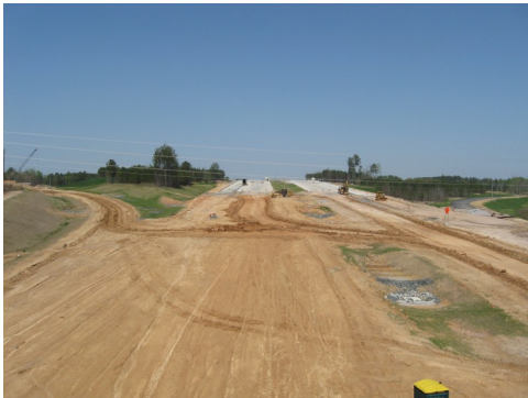
Construction of NC 540 as seen from the newly opened Beaver Creek Commons Drive (see next page for details).
